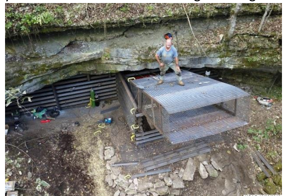
Drone view of Cobb Cave gate under construction. (Note the fish-plate arrows, to direct bats toward the new entrance.)
