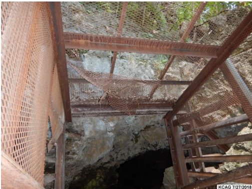
Breach at Lower Burnt Mill Cave
