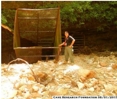
Damaged chute gate at River Cave after sinkhole collapse secondary to flood events. Before sinkhole collapse, this chute was ten feet above the sinkhole floor! Cooley is standing on a ten-foot-deep detritus field.
