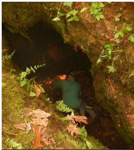
George Bilbrey welds up repairs on vandalized cave gate 14 feet below the surface at Lost Man Cave on the ONSR, Carter County.
